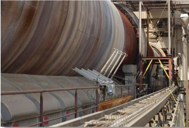
Figure 8: Cooling unit with four nozzles, four pyrometers and a controller
